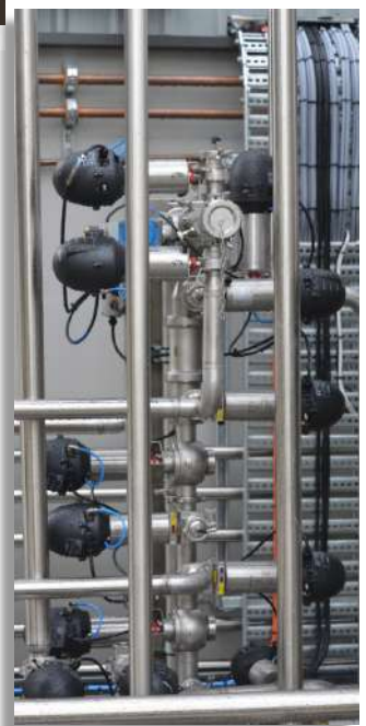
Designed and Installed complete process, incorporating a full product recovery system to maximise product yield and control effluent discharge.
